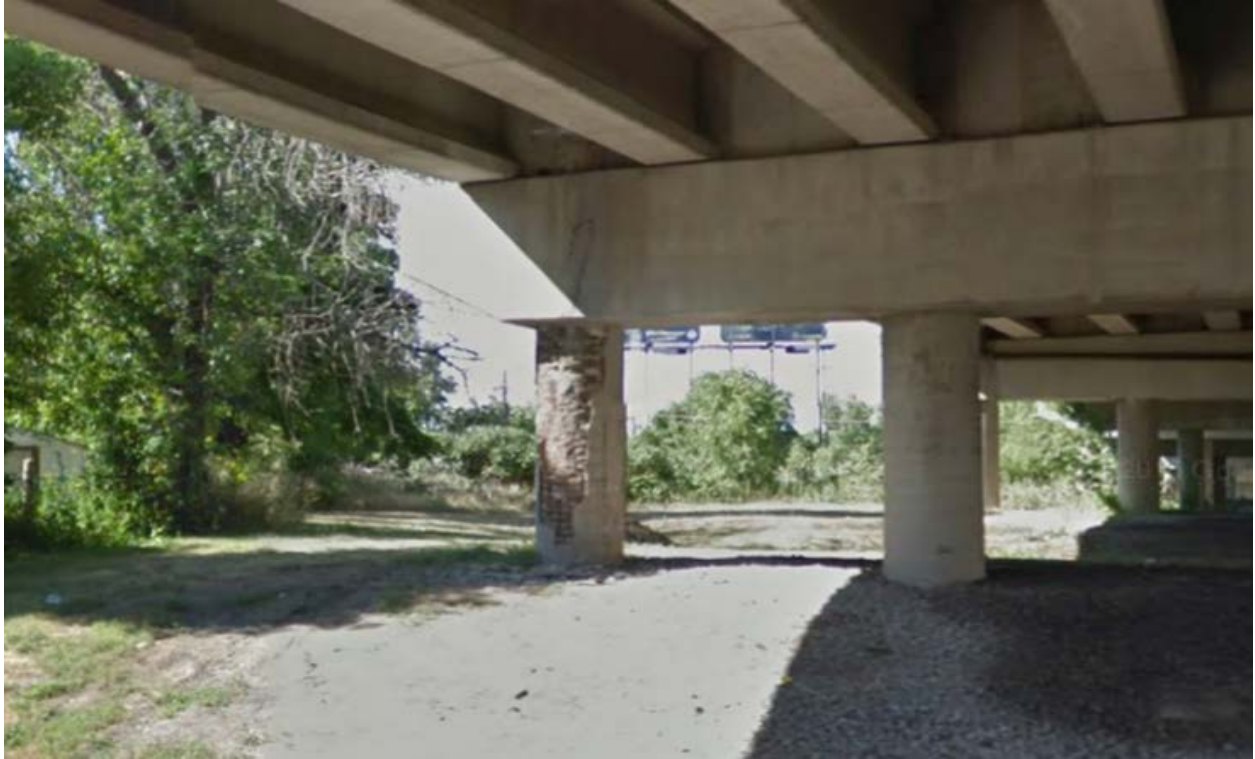
Above: Column in need of repair. Deteriorated concrete cover and corroded reinforcing is visible in 2012.
