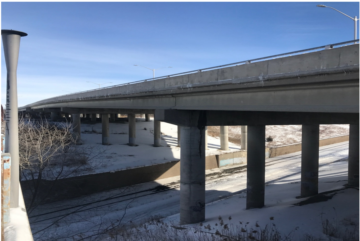
Columns repairs extremely close to CN Tracks which requires delays in work for passing trains
