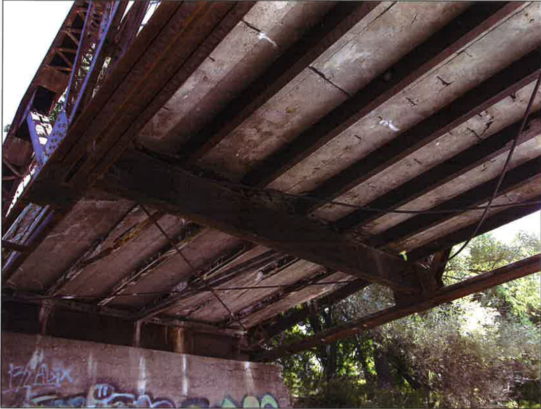
Deck Failure – East Bay
