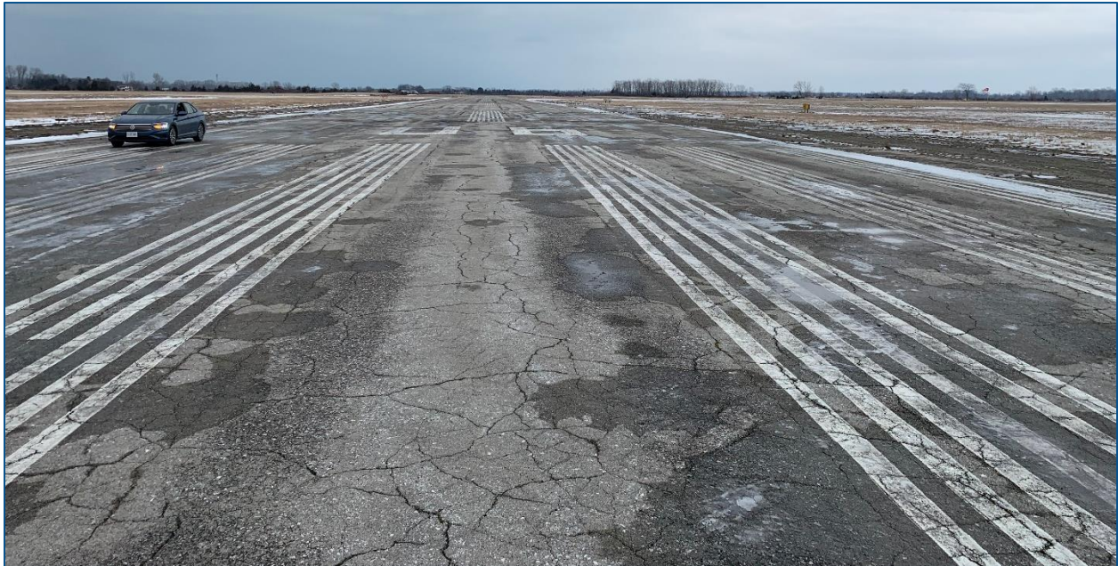
Runway 06 threshold and typical pavement distresses
