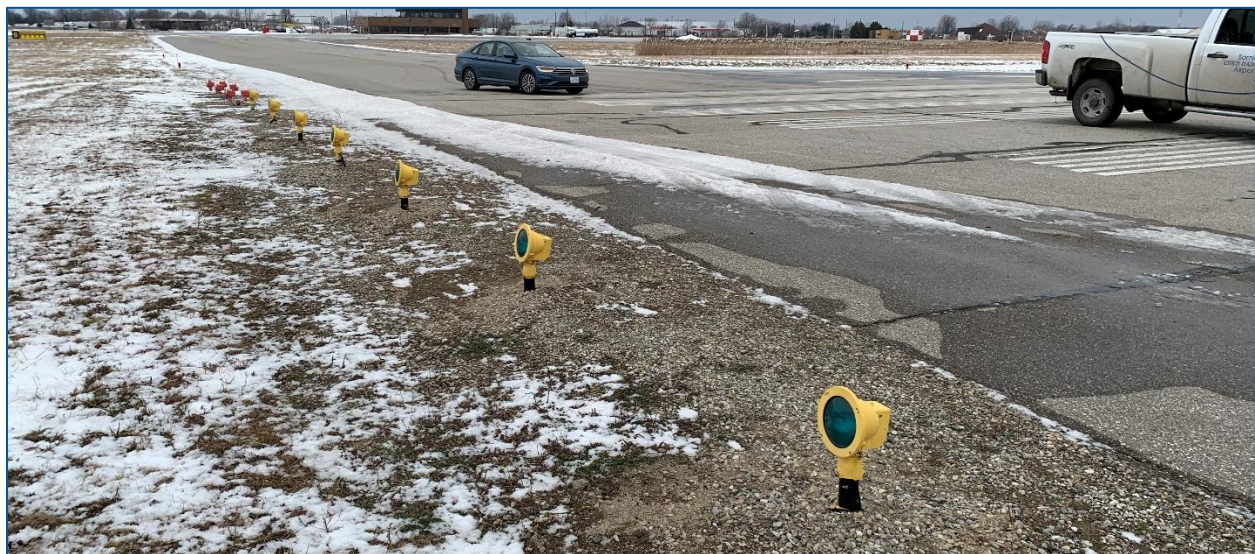
Runway 33 threshold lights
