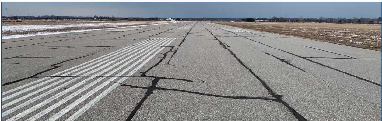
Runway 15-33, including typical longitudinal and transverse cracking
